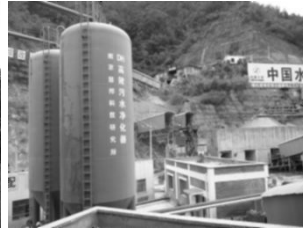
③ Production Wastewater Treatment
