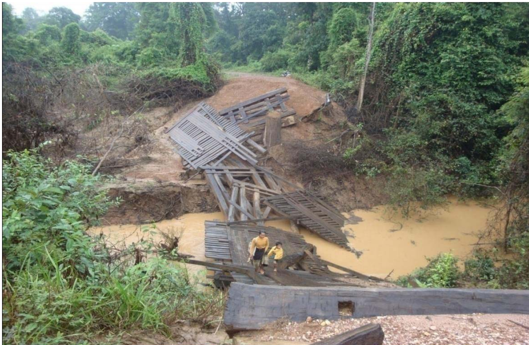
Figure 5.3: Post Ketsana: Loss of a bridge in the south of Lao PDR
